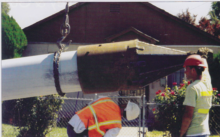
Of the entire 29,000 ft to be replaced in Phase 2 of the project, 22,000 ft was installed using pipe bursting.
