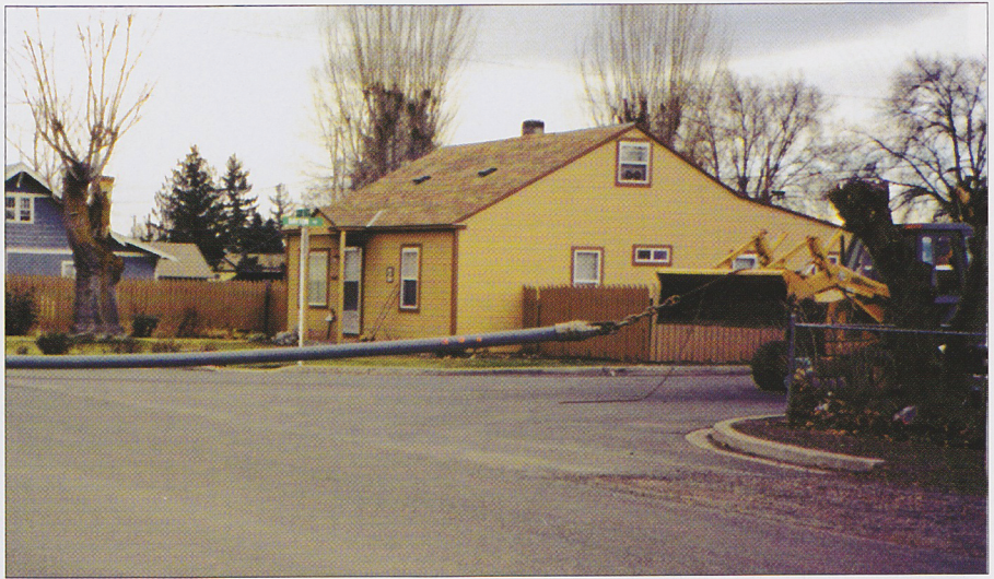
The six-man TTS Northwest crew began working in July 2003 through alleys since all the lines ran through residential and commercial areas.
